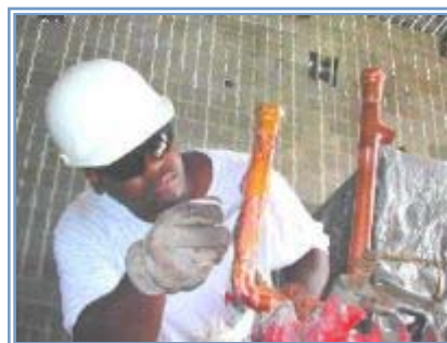
William Mitchell of W.W. Gay Mechanical Contractors welds copper tubing inside the new Arlington Middle School. --John Carter/staff
