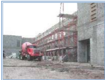
Phase One of the new Arlington Middle School is scheduled for completion by year's end. --John Carter/staff
